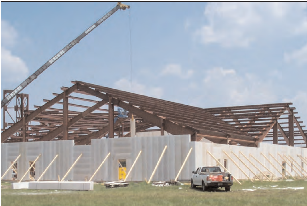
AERCON non-load bearing vertical wall panels connected to a steel frame structure.
