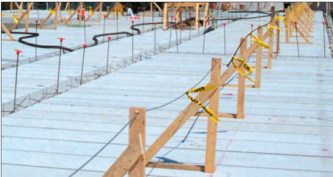
Reinforcing is placed in key joints between panels for continuity and diaphragm performance.
