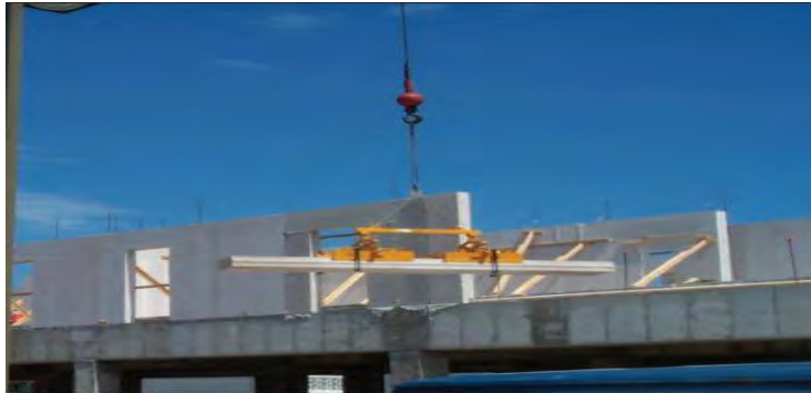
AERCON floor and roof panels are installed using a crane and clamp.
